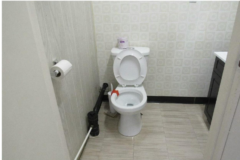
Photo #M7: Typical fixture in the Main Shop washrooms.
