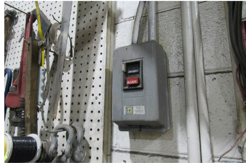
Photo #E6: Motor starter in the Main Shop.
