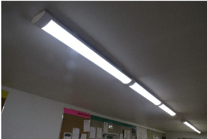
Photo #E9: Typical T-8 lighting fixtures, located in the Main Shop lunchroom.
