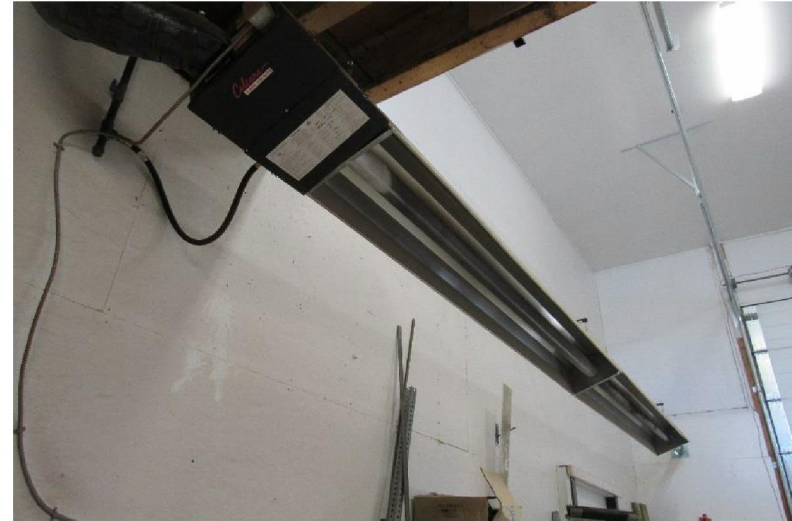
Photo #M10: Radiant heater found in the South Shop mini excavator loading bay.
