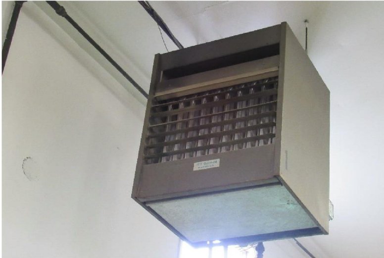
Photo #M9: Unit heater in the South Shop facility.
