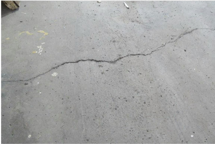
Photo #S1: Cracks on the SOG in the Main Shop.
