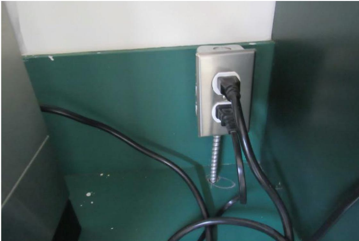
Photo #E7: Non GFCI receptacle by the break room sink.
