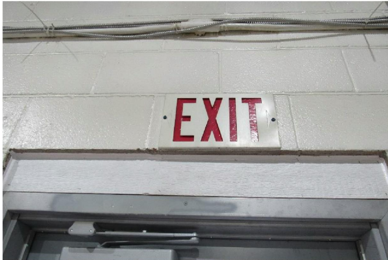
Photo #E3: Typical emergency exit lighting in the Main Shop.
