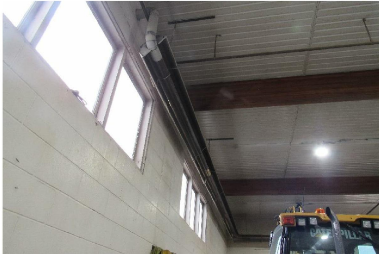
Photo #S3: General overview of the exposed metal roof decking and wood structure in the Main Shop.
