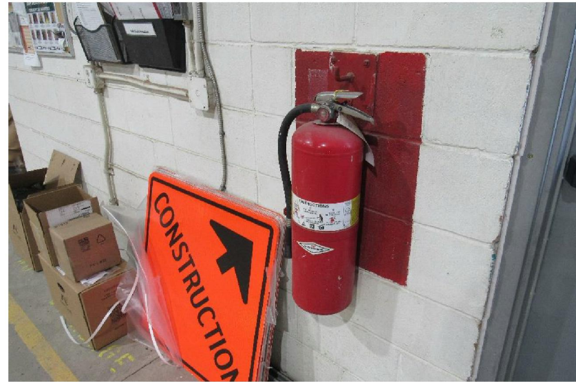
Photo #M4: Typical portable dry-type ABC fire extinguishers in the North Building.
