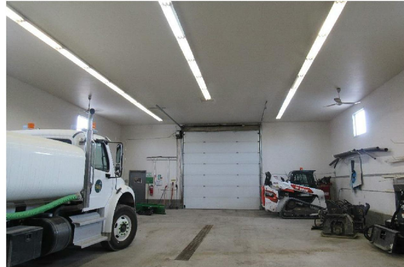
Photo #E10: Typical T-8 lighting fixtures of garbage truck loading bay, South Shop.
